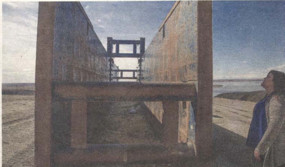
Shalee Russette, project manager for the Rocky Boy's/North Central Montana Regional Water System Project, stands beside a 60-foot long trench box that protects employees working on the pipeline.
