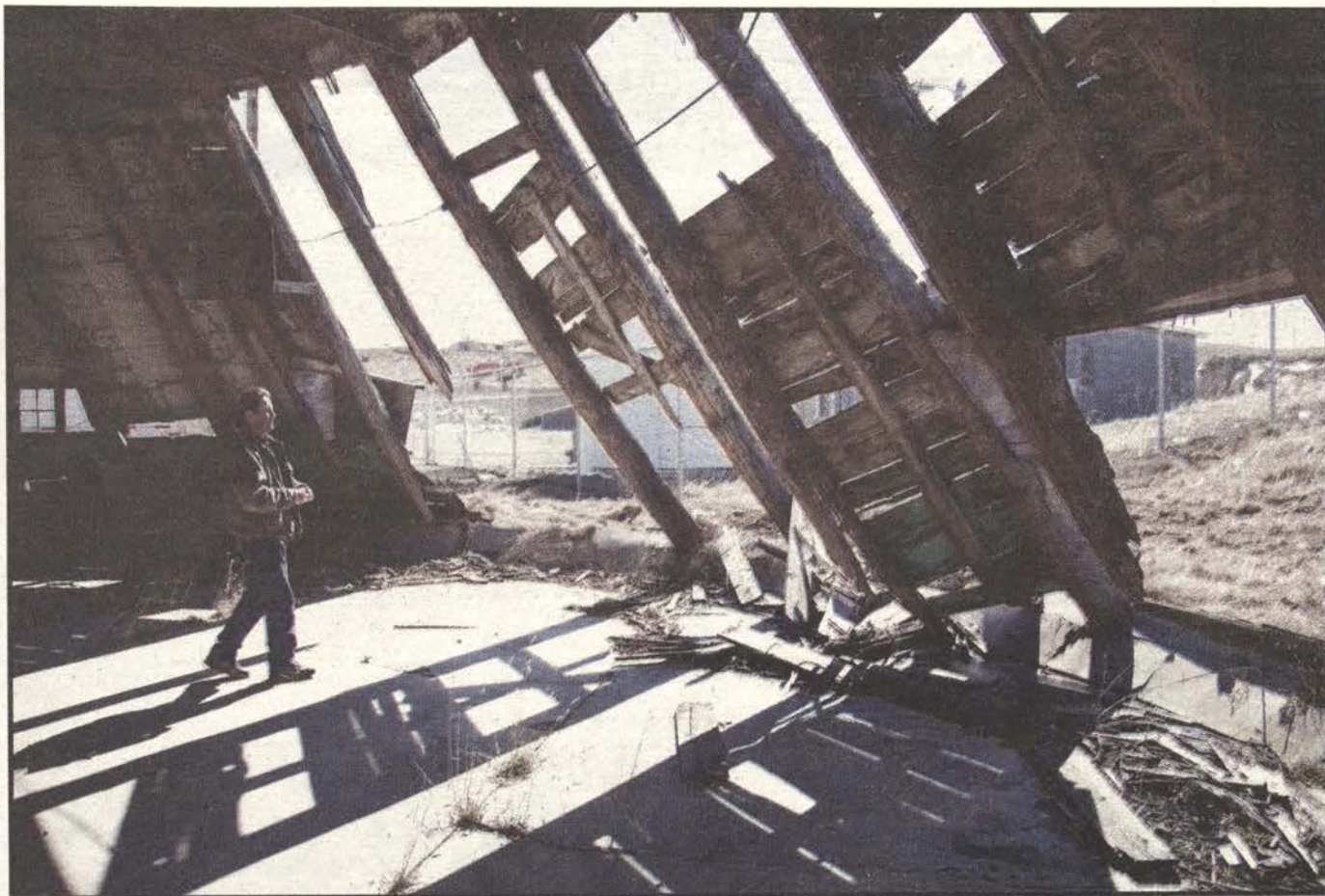
MAJOR ROBINSON talks about his plan to renovate a wooden teepee in Busby. "Maybe we will build a staircase along that wall up to the second floor, use the first floor as a story telling room and the second as a shop," he said. "We will paint it the colors of Northern Cheyenne: light blue for the people and burnt orange for the landscape."
