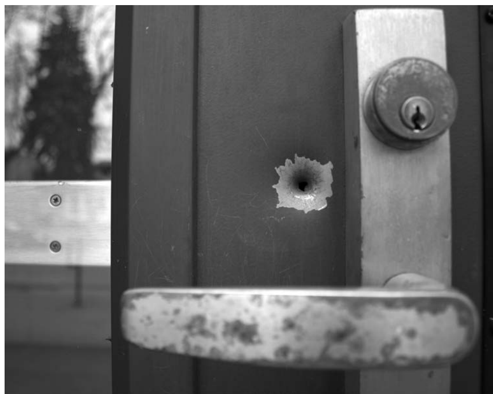
Several years ago the UCC was shot at in the middle of the night. The front doors and walls still show the bullet holes.
