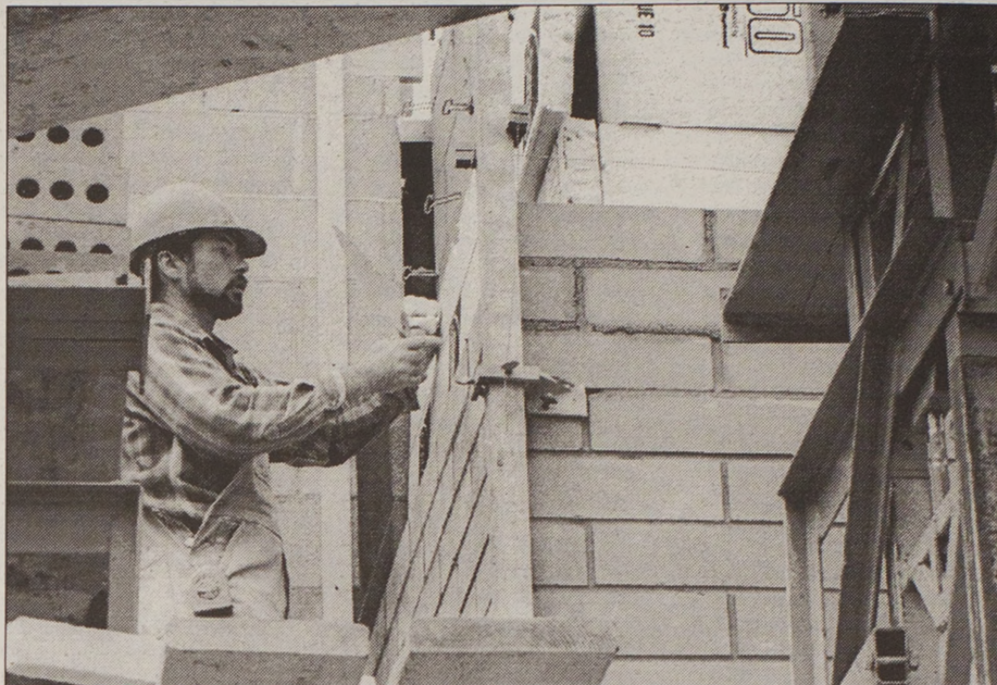
Jeff Jenne of Jenne Masonry stops to make sure the bricks he is laying are perfectly level for the archways of the east entrance into the new Recreation Annex Wednesday afternoon. Lisa Hornstein/Montana Kaimin
