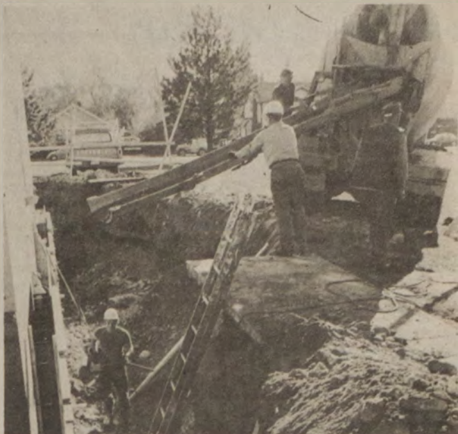
CONSTRUCTION workers are installing a stairwell and a fire exit on the west side of the Chemistry-Pharmacy Building to conform with federal regulations. (Staff photo by Mark Scharfenaker.)
