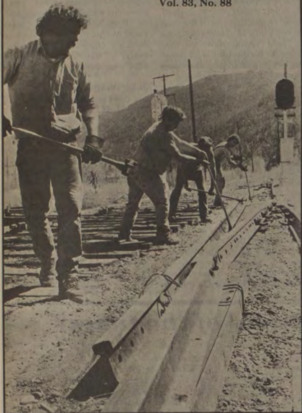
SAY GOODBYE TO the Milwaukee Road tracks, which are being ripped out here near the Van Buren Street footbridge. The A & K Materials Co. workers, who earn $3.50 an hour, are, from left: Kevin McDowell, Mike Woodward, "Dackfyl" Smith and Mark Savage. (Staff photo by Kinney.)
