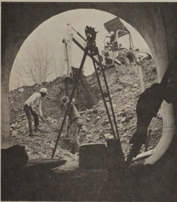
A WORM'S-EYE VIEW of construction of the new Van Buren Street Bridge Underpass is shown above. The pedestrian and bicycle underpass is being built across from the Harry Adams Field House on the northwest edge of campus. (Montana Kaimin photo by Tom Levno)
