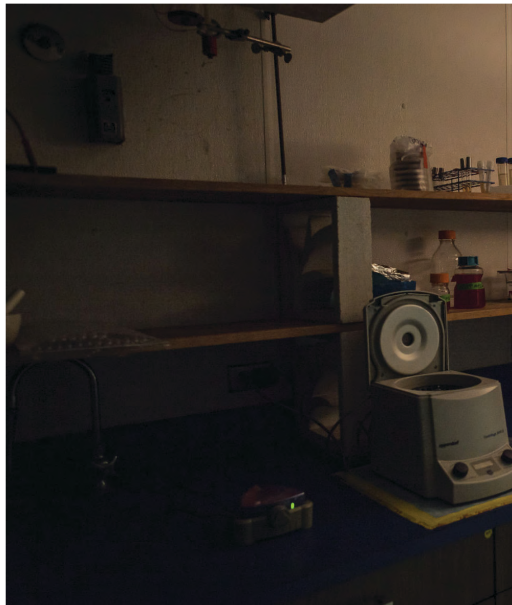
A floor lamp illuminates a walk-in cooler in a second floor lab in the Charles H. Clapp building at the University of Montana, highlighting the presence of asbestos in the ceiling.
