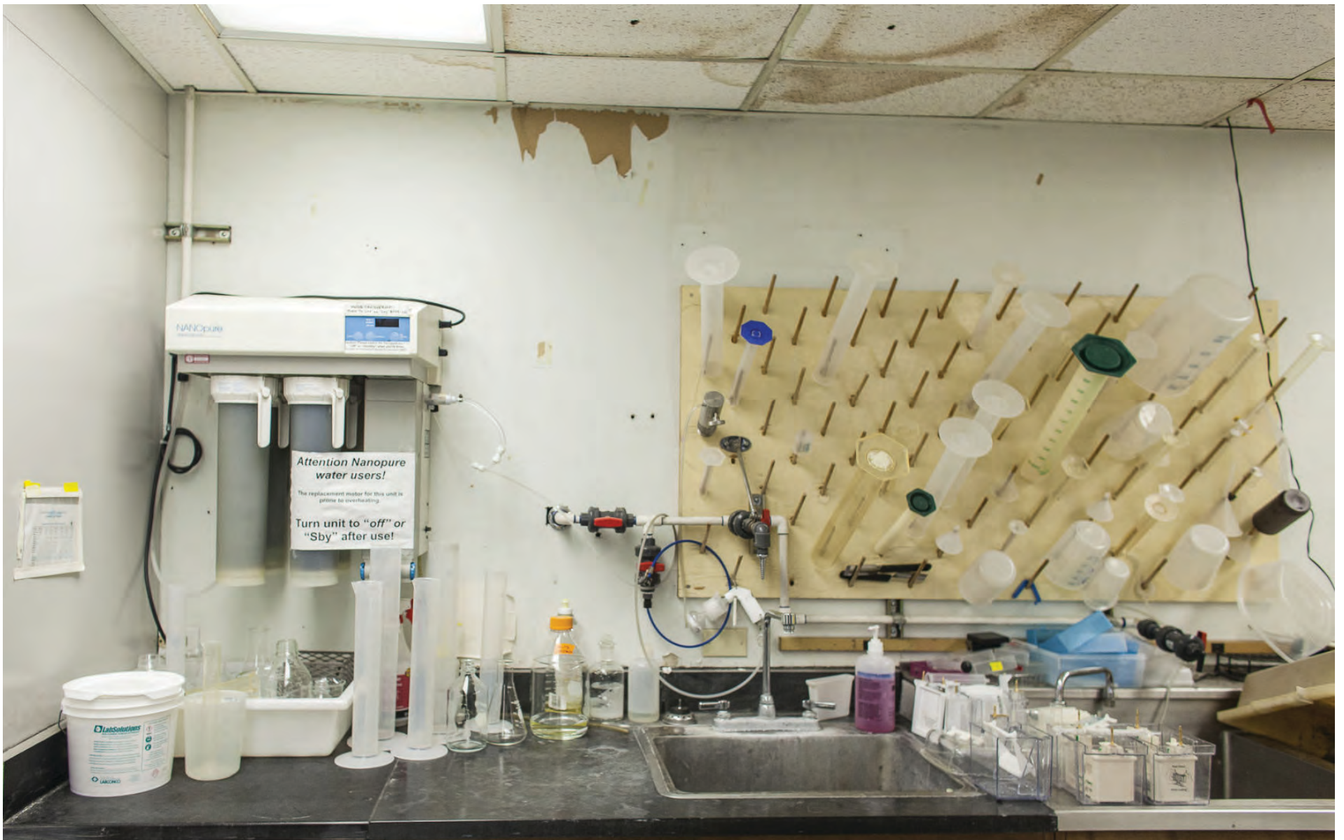
Damaged ceilings and walls in a lab on the second floor of the Charles H. Clapp building at the University of Montana. The damaged tiles are the only thing keeping asbestos in the ceiling.
