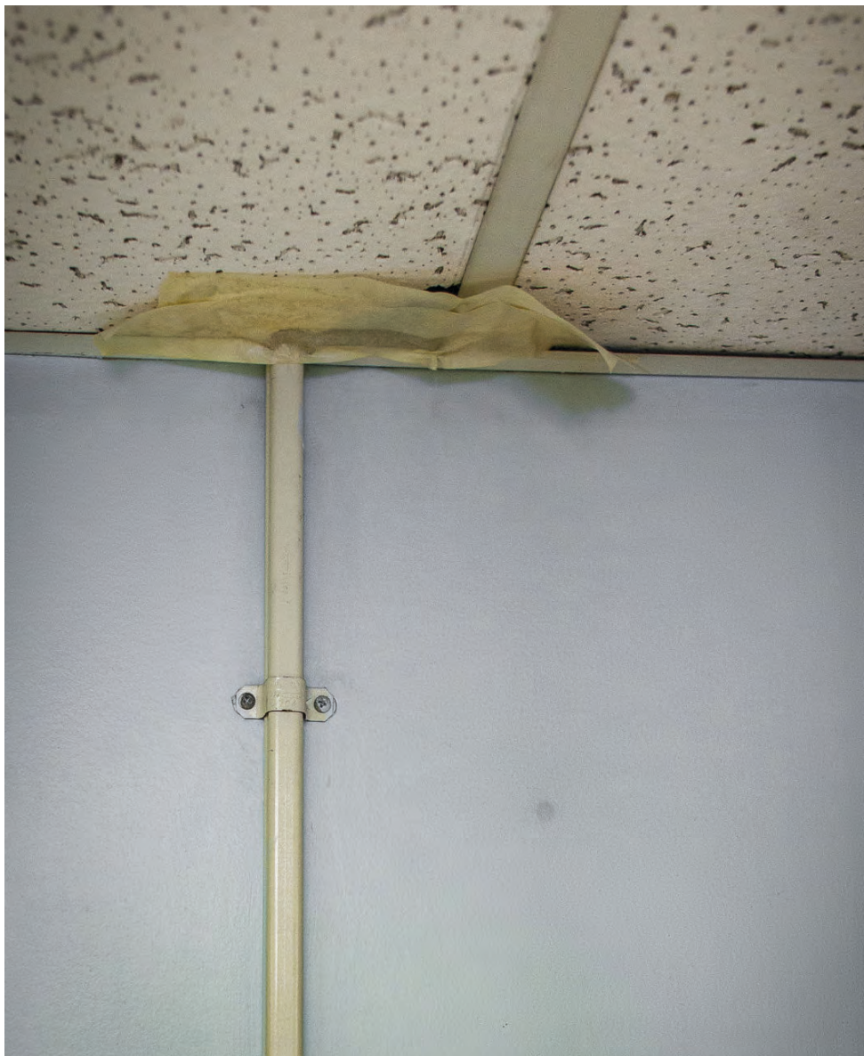
Masking tape peels away from where it was placed to cover a hole in the ceiling, supposedly to protect from asbestos in the ceiling.
