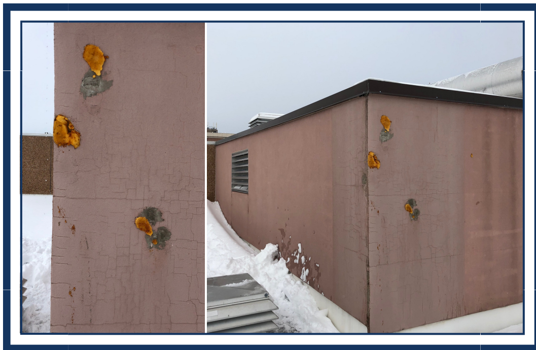
Figure 17. Penthouse mechanical room woodpecker damage
