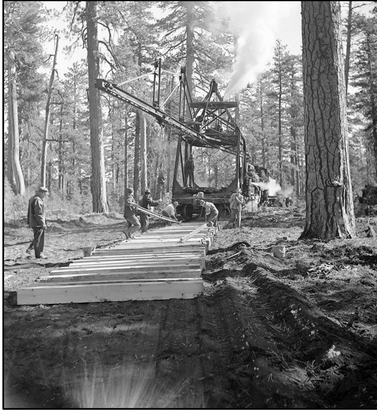
Figure 8. Track Laying for the Fruit Growers Supply Railroad in 1946 at Halls Flat, California. Image courtesy of University of Montana, Mansfield Library, Archives and Special Collections, Phillip C. Johnson Collection: Photo number 92.1874. (As of 12-26-2019, this photo was not in the Montana Memory Project collection.)
