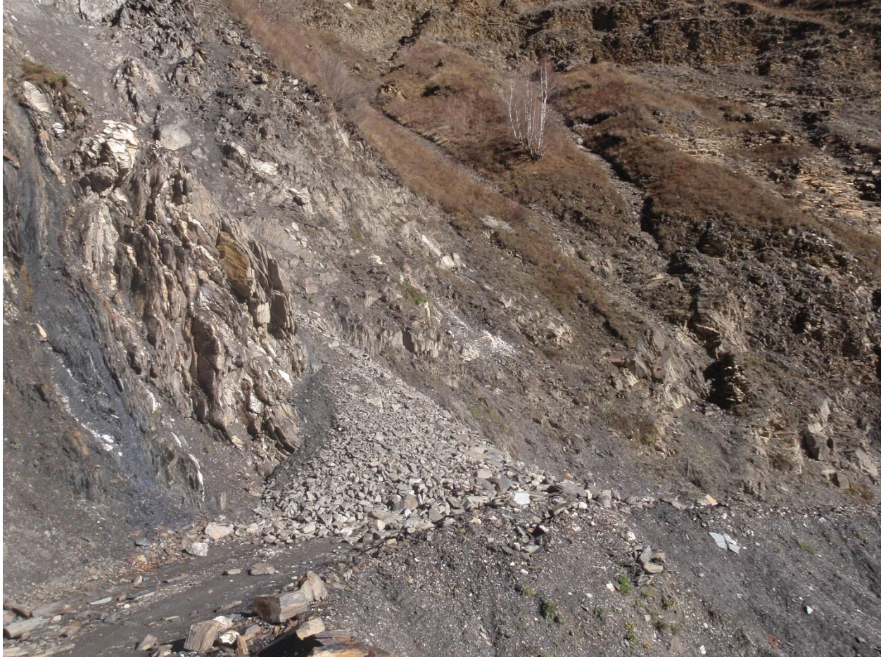
Figure 8 The narrow stretch of road between Ushguli to Kala is most affected by debris and avalanche flows, requiring assistance from tractors to keep clear. The old Soviet-era machines are operated and maintained entirely by locals. The closest source of fuel is in Mestia, and the tractors are prone to mechanical failure and snow storms and other geohazards can stop vehicle traffic for days to weeks (Photo by Peter Bordokoff, November 2012).
