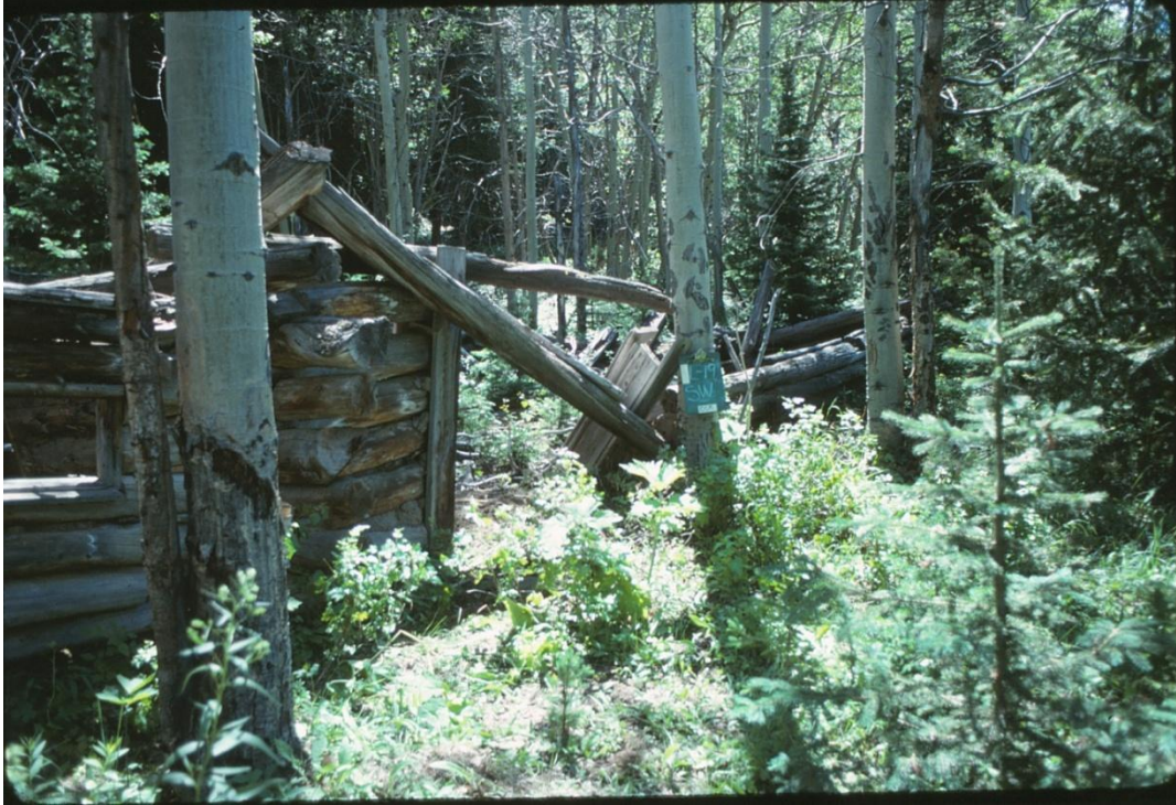
Figure 4.13. Showing the SW elevation of building at Locality 19 and the division between the two rooms of the structure (German Gulch Paperwork Archive, GCM 1989).
