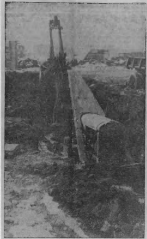
Actual construction of the art museum-lecture hall building on the State University campus, to face on Maurice avenue, got under way Monday morning, when the big shovel shown above dug out the first bucketfull of dirt and then proceeded rapidly with the excavating.
