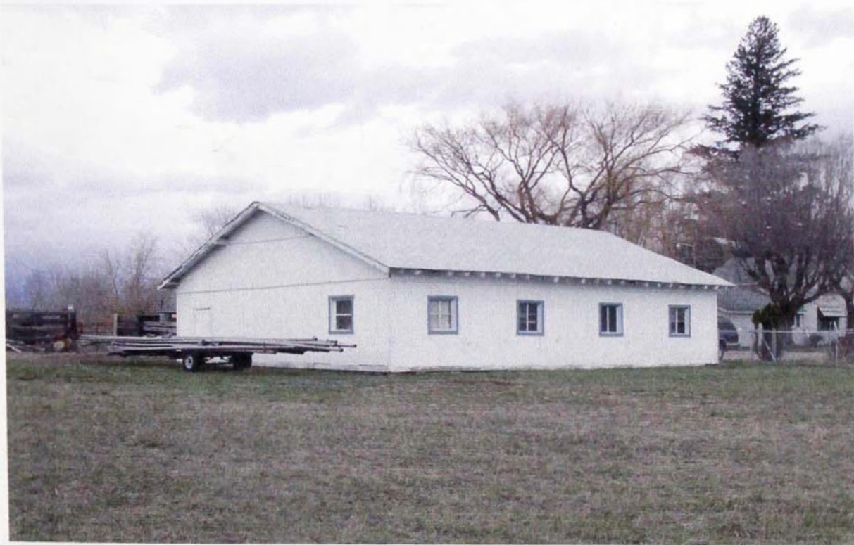
Figure S12 – View of the southwest corner of the equipment barn, looking northeast; wood corral feature on left; main house on right.
