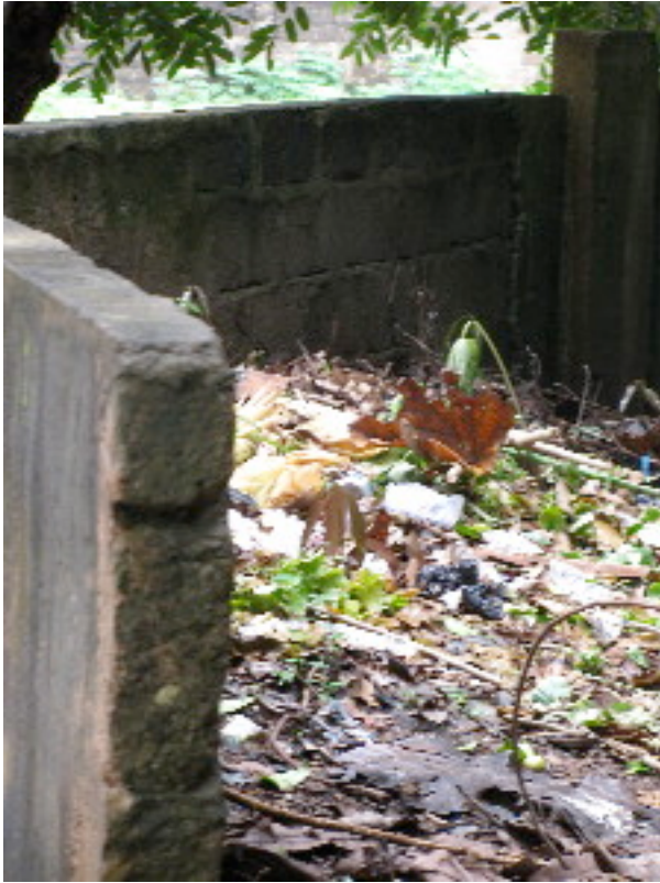
Figure 26. Rubbish behind the wall in Figure 24
