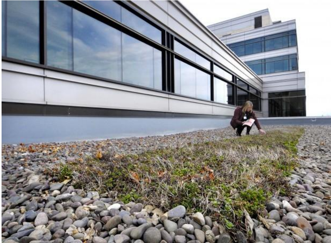
Figure 3: A demonstration extensive green roof sedum strip atop St. Patrick Hospital, Missoula. Photo via www.missoulian.com .
