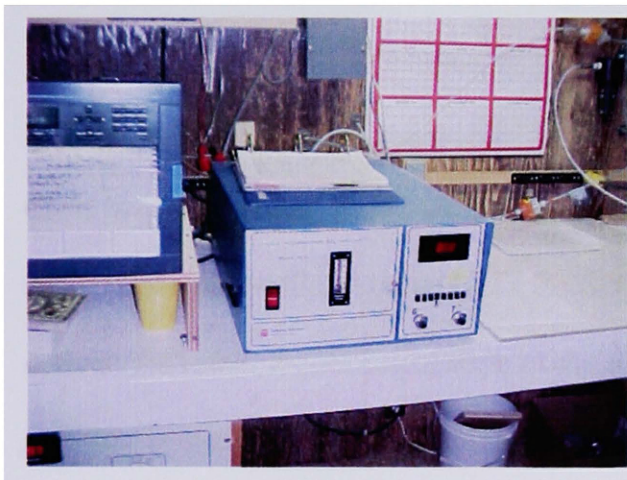
Figure 3-3 H_2S Analyzer (Ambient Site 2)
