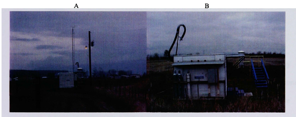
Figure 3-2 Ambient Stations (A) 1A (Mocassin Lane), (B) 2 (# 2 Well Field)
