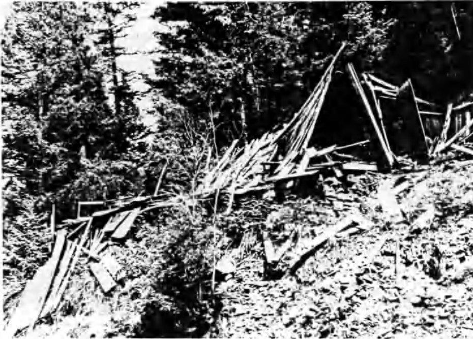
Figure 46: A building near the Mussingbrod mill. Notice that the structure has completely collapsed upon itself and prevents any visual investigation of the floor
