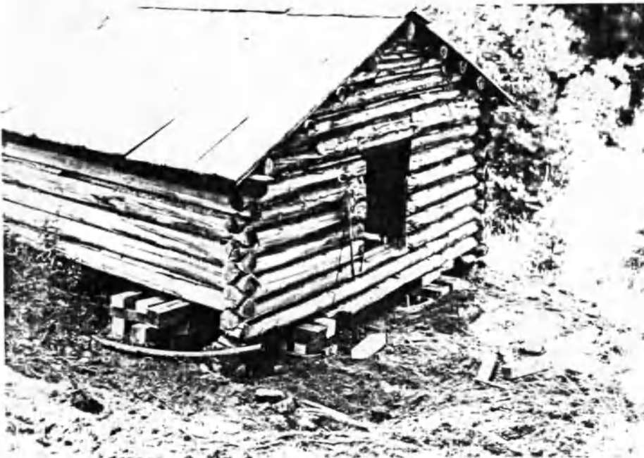
Figure 101: Another view of restoration and stabilization in action. None of the dirt that the backhoe has removed was screened for material culture (personal observation, 1993).
