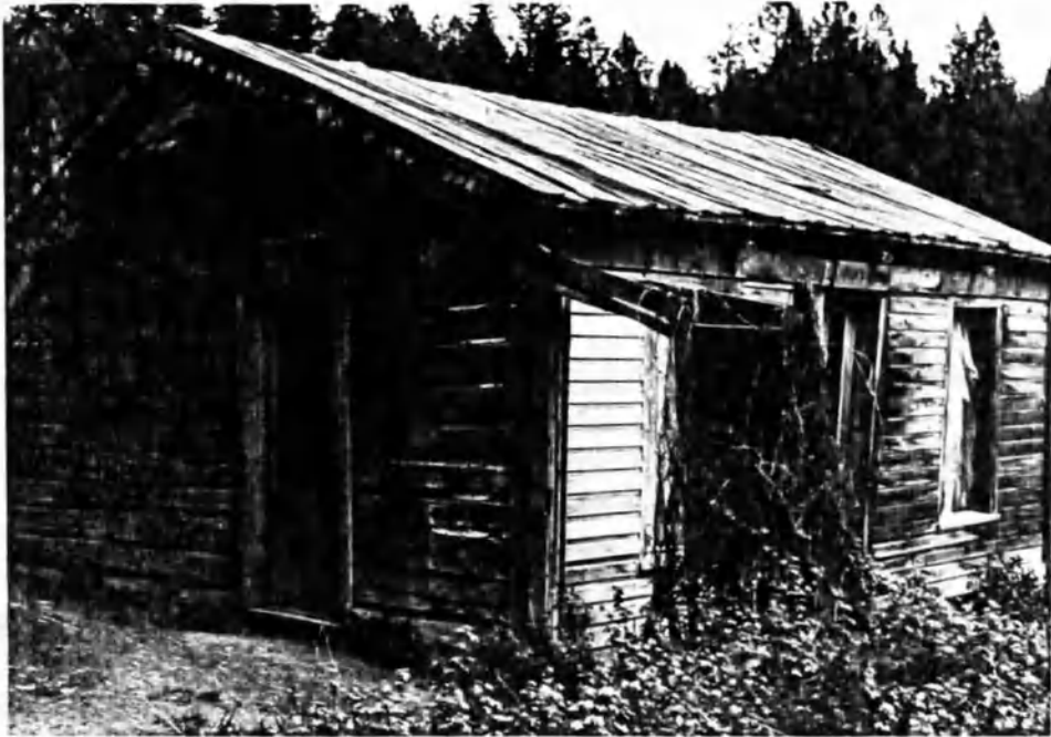
Figure 18: A 1994 photograph of the Adams family house. Notice the repair of the roof and that the walls are upright, not sagging in the middle, as seen in Figure 17
