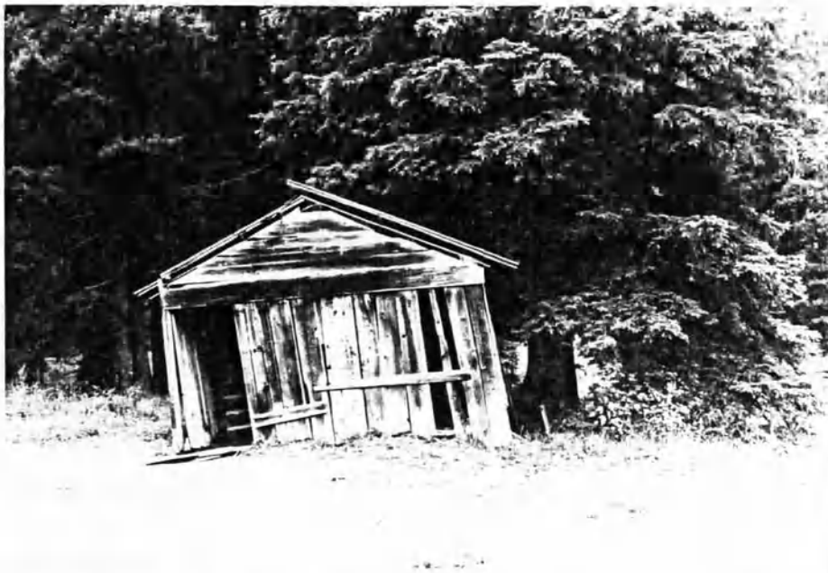
Figure 91 This cabin has only two small windows. There is no foundation which is seen by the tilting of the structure.
