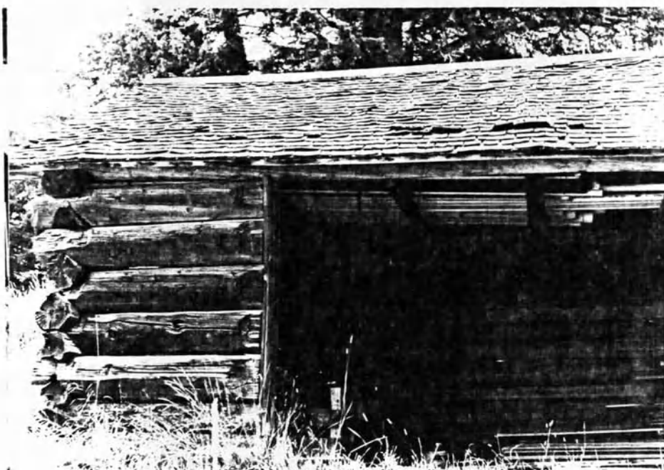
Figure 106: A photograph of the shed just south of the Hannifen house. Originally this was a cabin, but the structure's abandonment left it available for others reuse or salvage.
