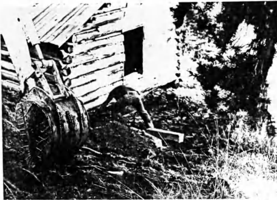
Figure 100: A view of restoration in action at Garnet. The backhoe was used to remove excess dirt surrounding the cabin and facilitate the installment of a drainage field.
