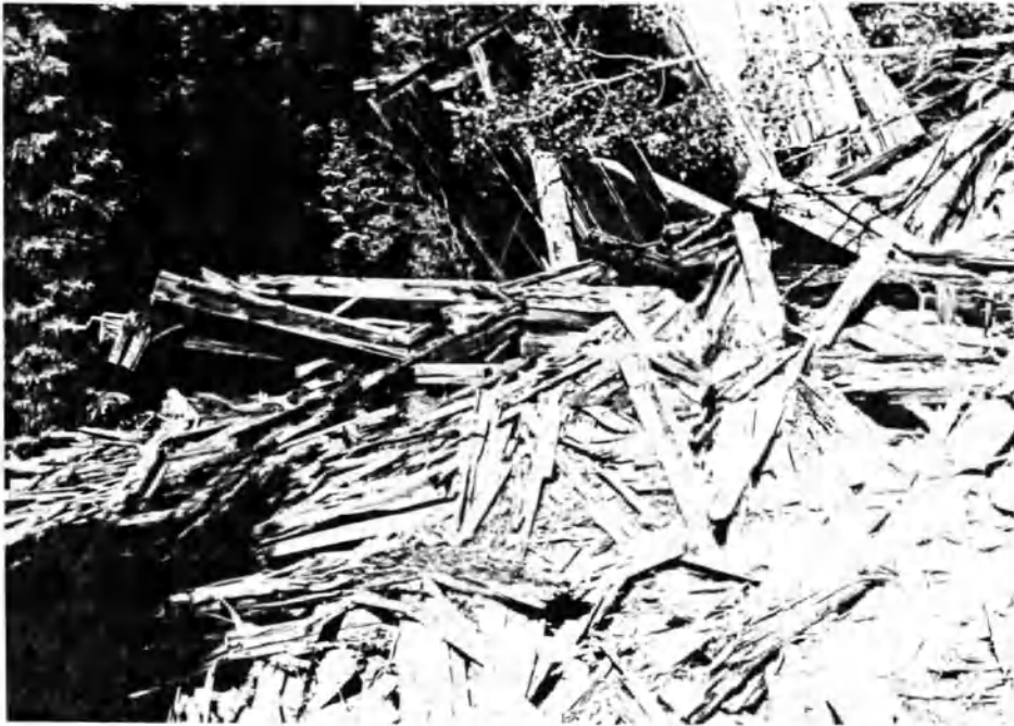
Figure 88: A photograph documenting the results of continued years of environmental processes at work. This section of the Mussingbrod mill has collapsed upon itself preventing any documenting of refuse concentrations.
