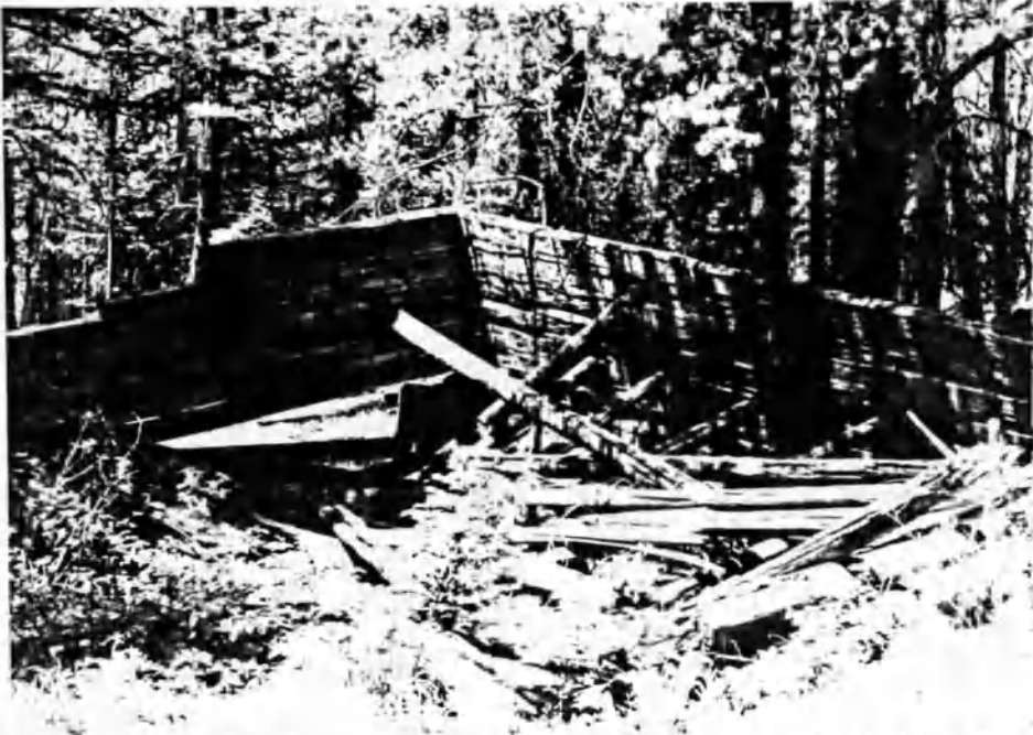
Figure 48: A photograph of the alleged location of the brothel. The roof has collapsed in upon itself.
