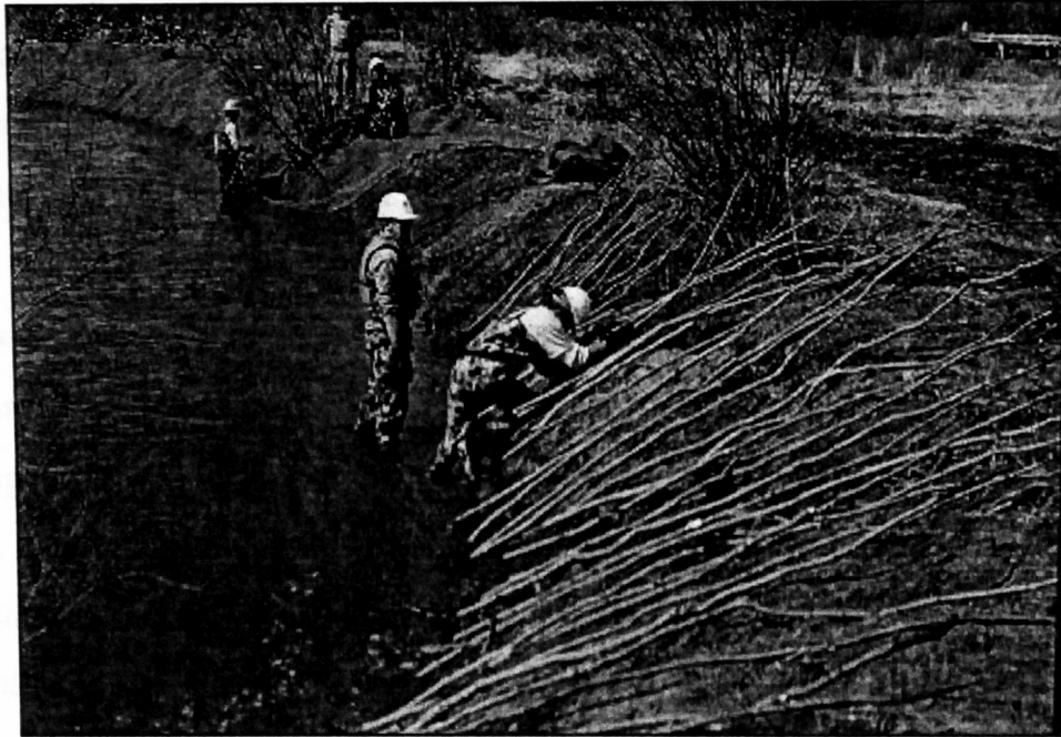
Figure 6. Placement of angled Salix spp. cuttings along a re-sloped bank. Cuttings are approximately 3 m (10 ft) long and spaced at 30 cm (1 ft).
