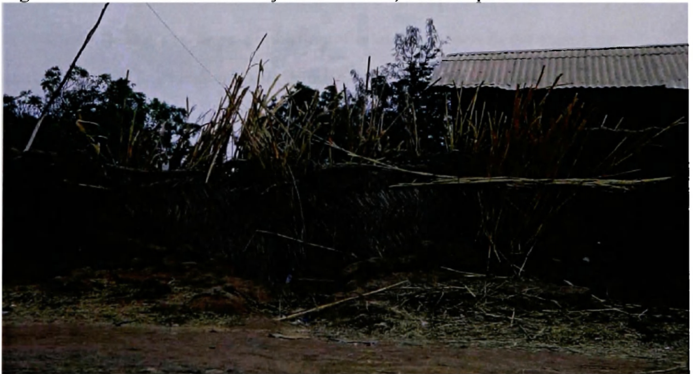
Figure 2- A wall knocked down by wind and rain, and then patched
