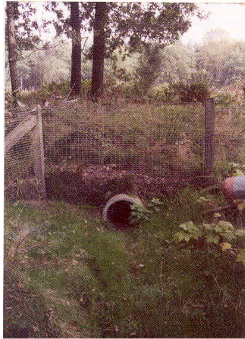
Figure A-3. Smaller mesh fence. Note potential problem with litter build up and fence not connected to outer edge of culvert. Photo: Bank et al. 2002.
