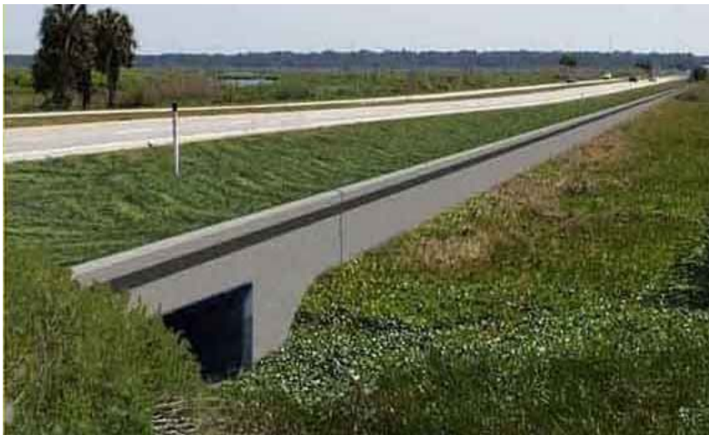
Figure A-7. Paynes Prairie Ecopassage (Florida) – Artist rendition. Concrete wall with lip. Photo: D. Forsyth. www.fhwa.dot.gov/environment/wildlifecrossings/amphibian.htm
