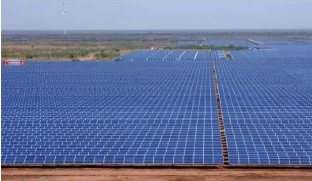
Figure 1: a view of Charanka Solar Park, Gujarat (source: first author)
