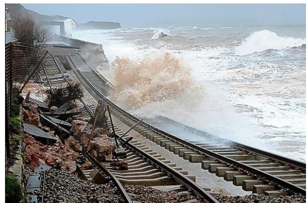
Figure 9: The main railway line to Cornwall and Devon was demolished at Dawlish by storms which hit the UK in February 2014 [15]
