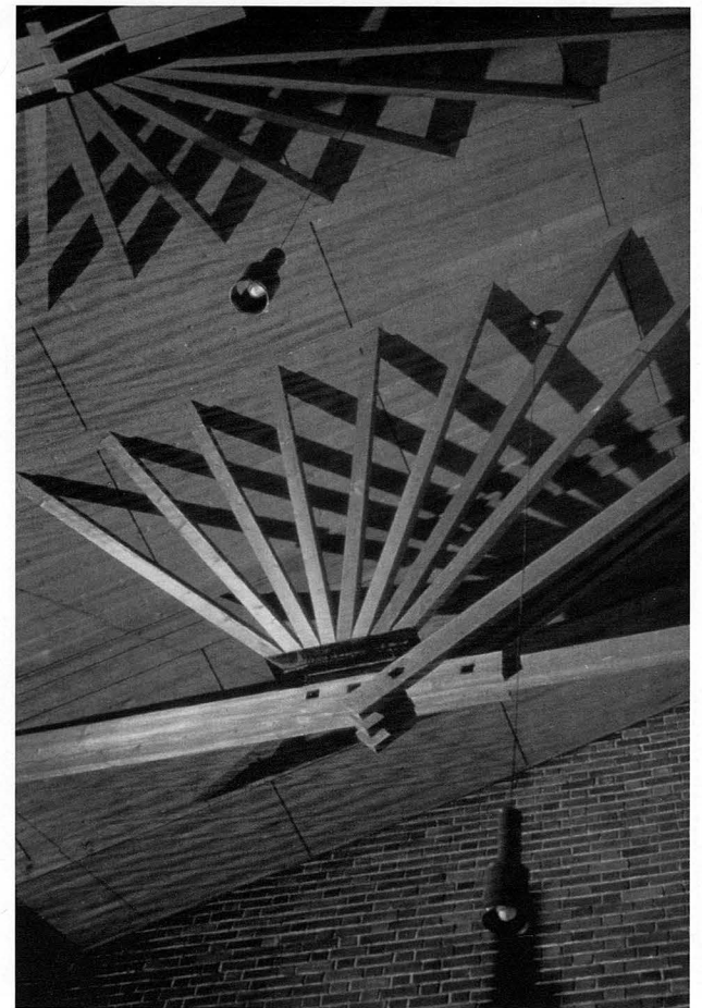
Distantly biomorphic imagery of the roof trusses of the Council Chamber, Town Hall, Saynatsalo. Photo Courtesy of the Museum of Finnish Architecture.
