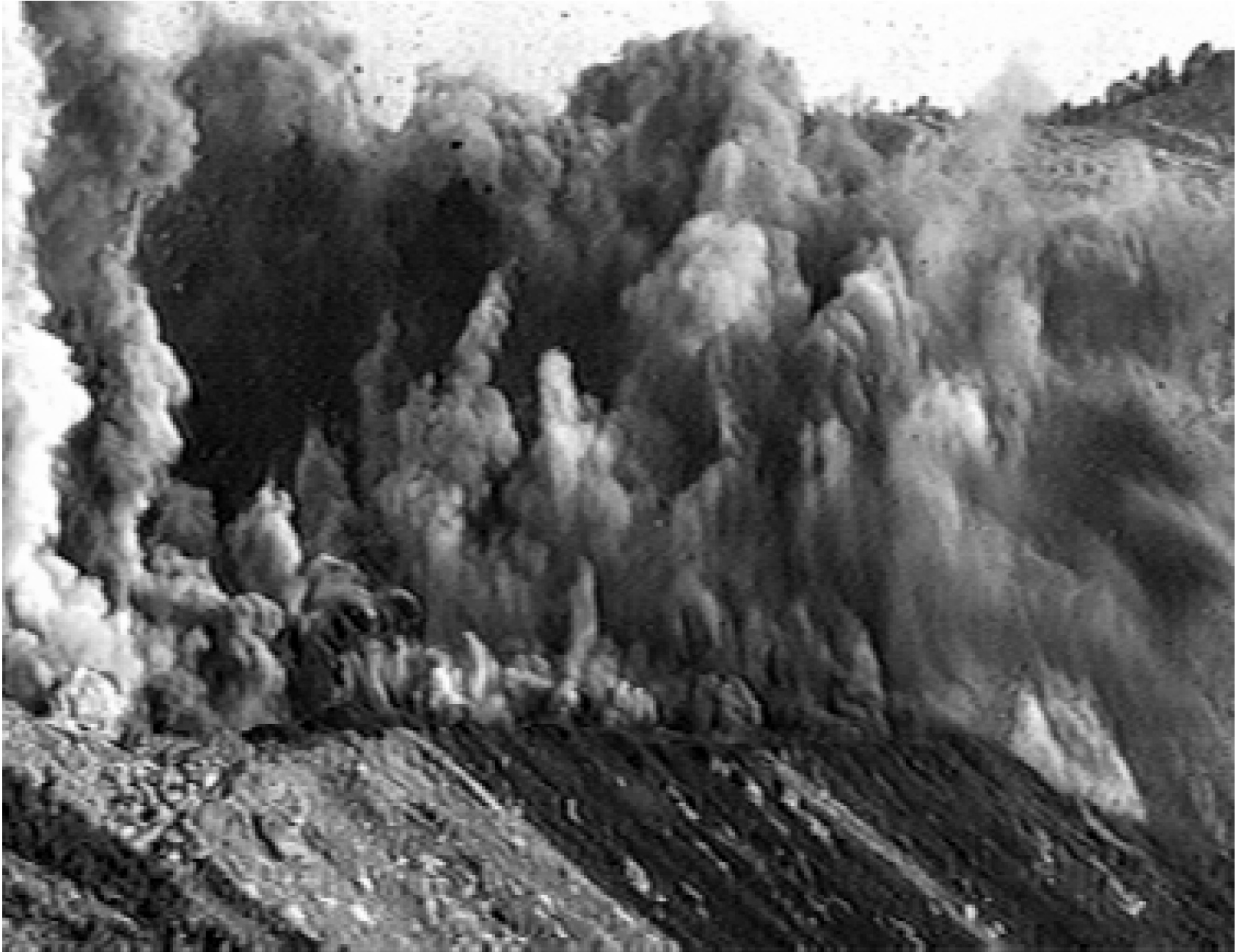
Fig. 4: Demolition charges used to remove a mountain ridge to establish faster Internet communications infrastructure between New York and Chicago.
