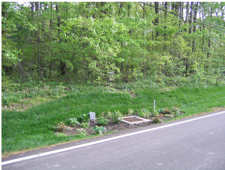
Figure 3. A bioswale was installed at this location in Orange Village (a suburb of Cleveland OH, USA) to expand infiltration opportunities for excess stormwater runoff generated by roads, nearby residential development, and legacy drainage issues. A catch basin was installed in the center of the bioswale run wherein monitoring gear is installed among the attractive horticultural plantings.
