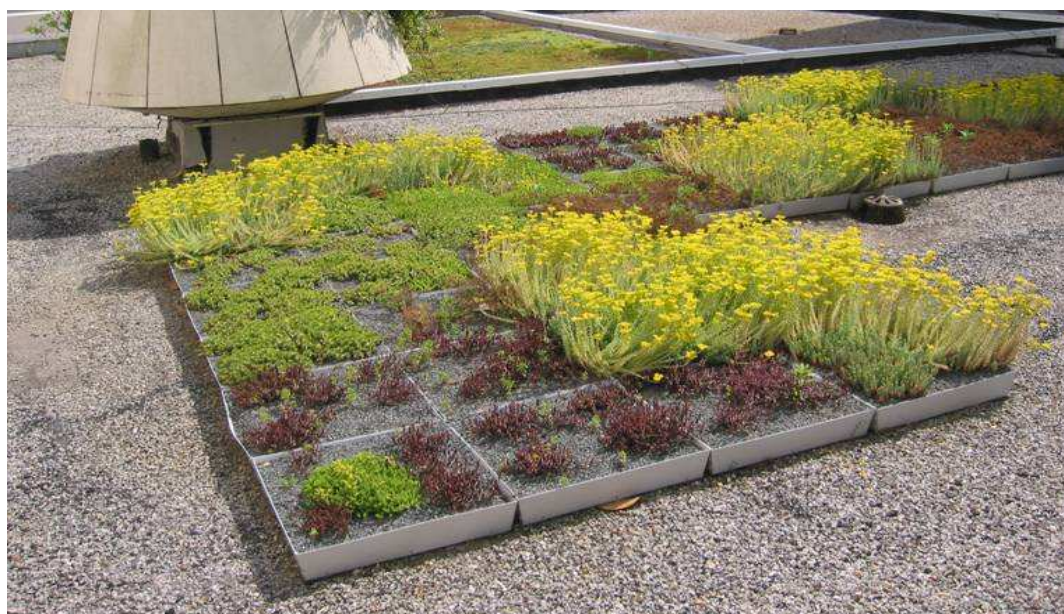
Figure 2. UGA modular green roof system.
