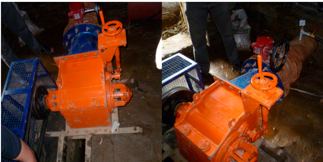
Figure 21. 5 kW Nepali-made Crossflow turbine (Photo credit: Sam Williamson).
