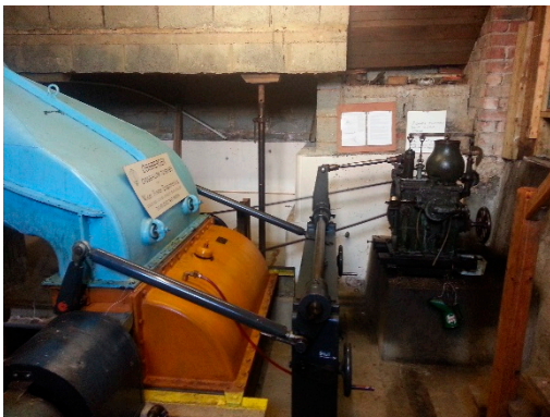
Figure 4. Ossberger Crossflow turbine with draft tube installation in UK (Photo credit: Sam Williamson).
