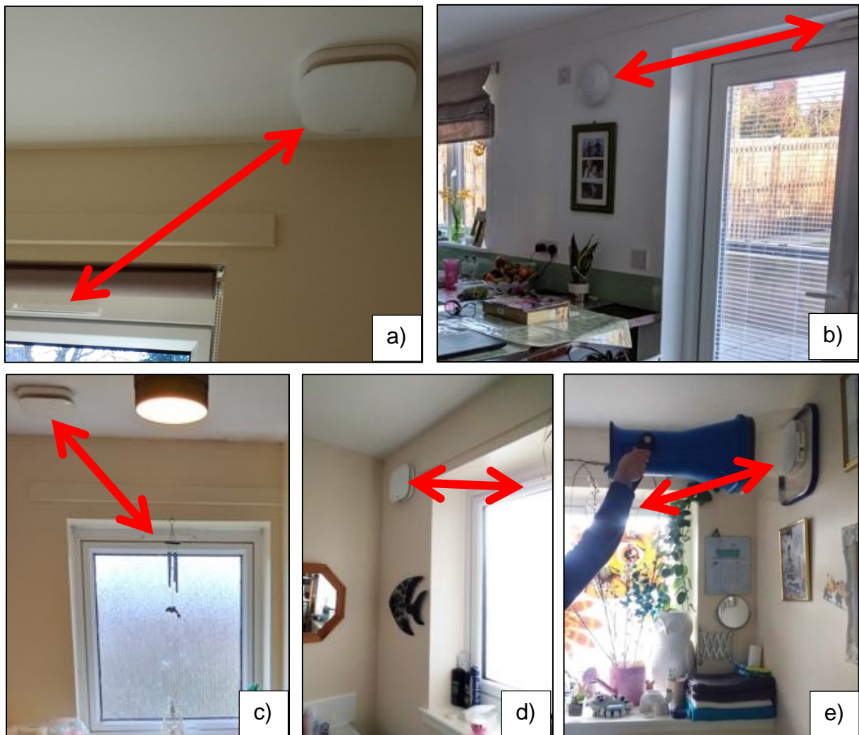
Figure 32. Examples of short circuiting, a) M21 Kitchen, b) M20 Kitchen c) M19 Bathroom d) M17 Bathroom e) M18 Bathroom
