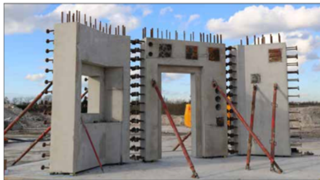
Figure II.5. Test assembly of precast RC solid solutions using headed bar joints for NPP applications [124].
