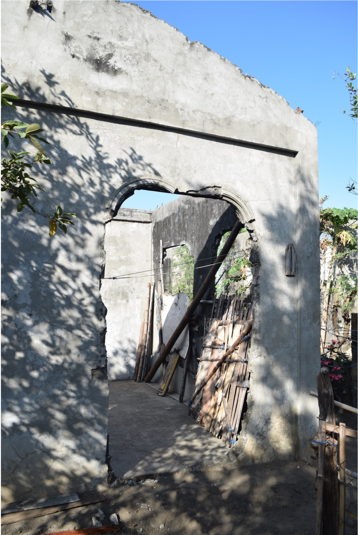
(Figure 11: Master weaver Mam Talin's typhoon damaged home. Credit Kelly 2019)
