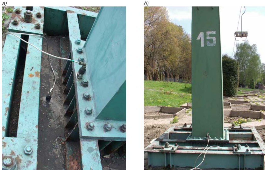
Fig. 4. A layout of sensors on tested elements: a) detailed view, b) overall view.
