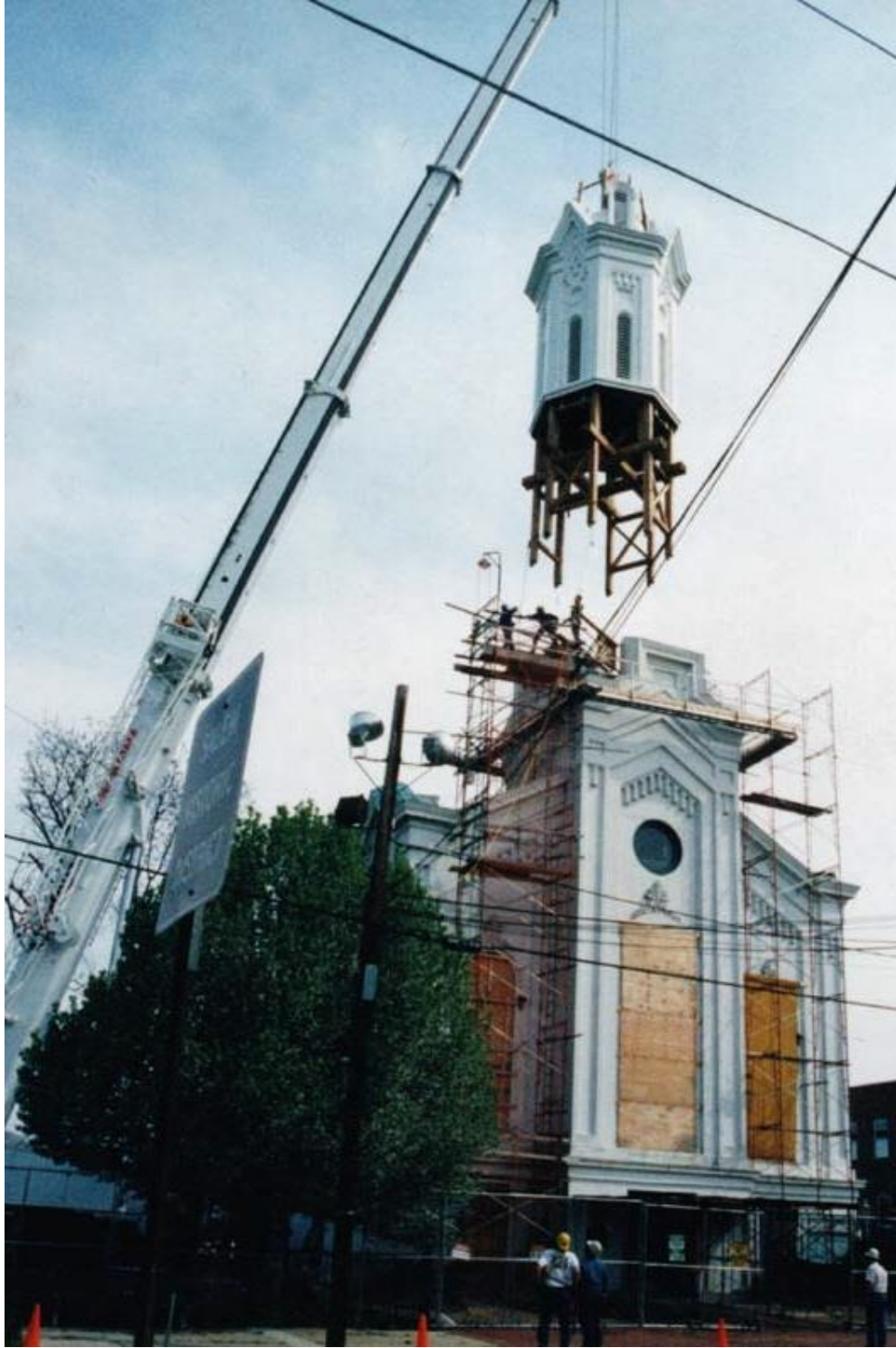
Fig. 29. Resetting of belfry frame, First Presbyterian Church, Salem, NJ (1997). Note scale of timber frame in relation to people on top of scaffolding. (Courtesy of Janet Sheridan.)
