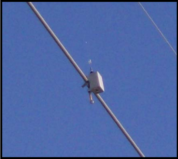
Figure 19. Typical BSI sensor installed on a 115 kV conductor during 2007 field tests
