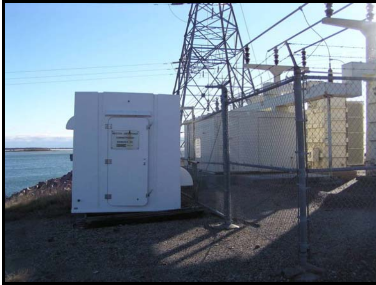
Figure 6. Communication shack housing the BSI base station
