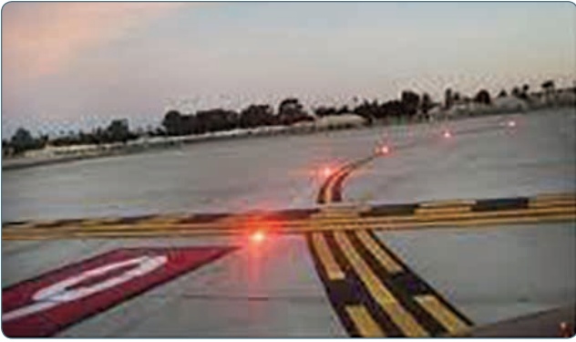
Figure 14-35. Runway Entrance Lights (REL).
