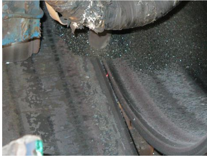
Figure 1.12: Internal welding of the SWP where laser-controlled seam tracking system used [NPC]
