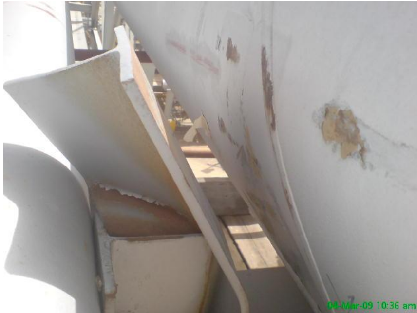
Figure 1.3. Mechanical damage due to pipe movement. (Courtesy, Saudi Aramco)
