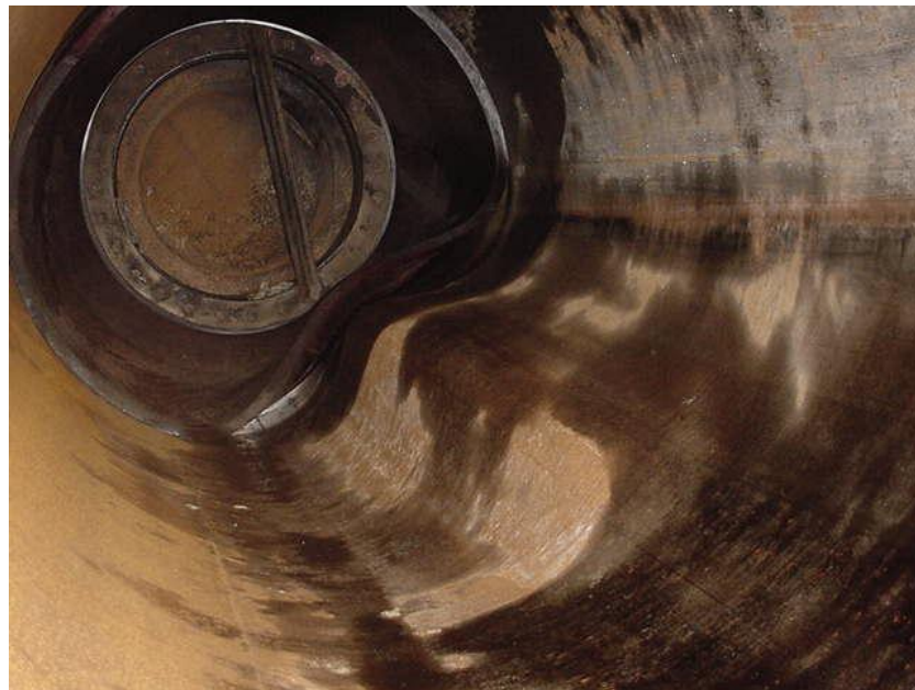
Figure 1.4. Pipe collapse under sleeve because of hydrogen trap. Shown also is a stuck pipeline scraper. (Courtesy, Saudi Aramco)
