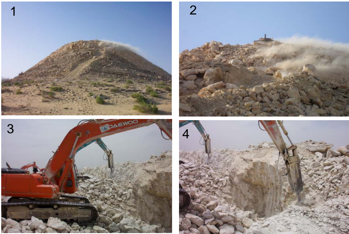
Figure1.8. Four photographs showing the removal process for Jabal Midra Al-Janubi by a local land developer during the year 2004.
