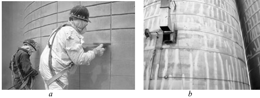
Fig. 9 – Strengthening solutions for RC silos: a – near surface mounted composite strips; b – carbon fibre composite hoop strips.
