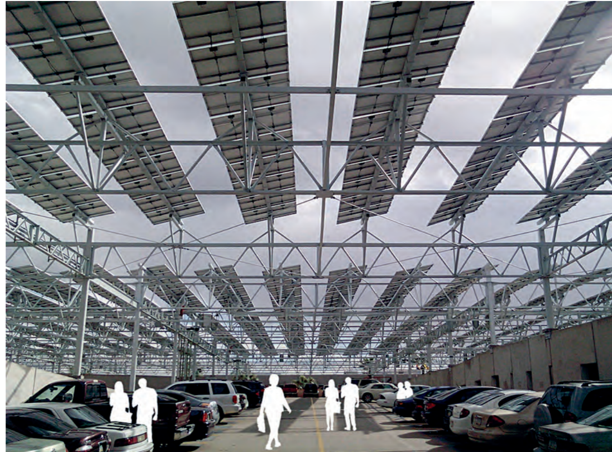
Parking facility-solar recharging station
