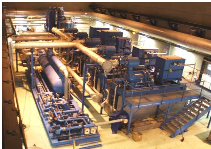
Figure 3 Compressor station of 18 kW @ 4.5 K cryogenic refrigerator
