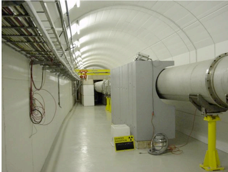
Figure 5.1: View of the additional Shielding installed after the Target Area.
