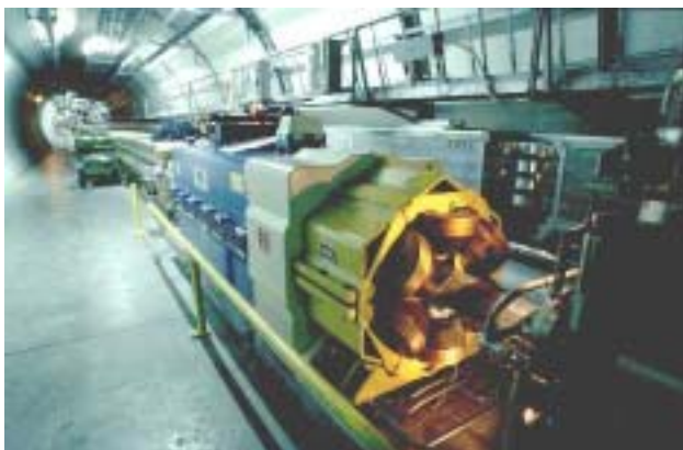
(a) Regular arc with sextupole/quadrupole assembly in the foreground
