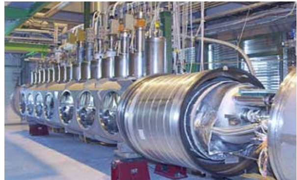
Figure 1 String 2 Electrical Distribution Feed Box
