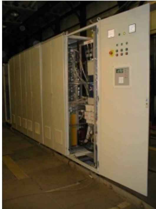
Fig. 6 View of completed cabinets of the SMES Modulator
