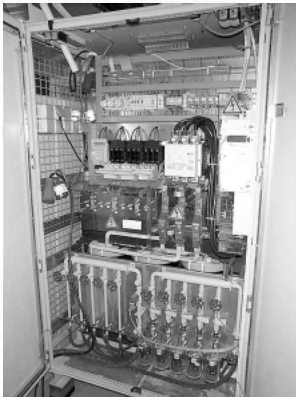
Figure 7: rear side of 300 kW switch mode power supply
