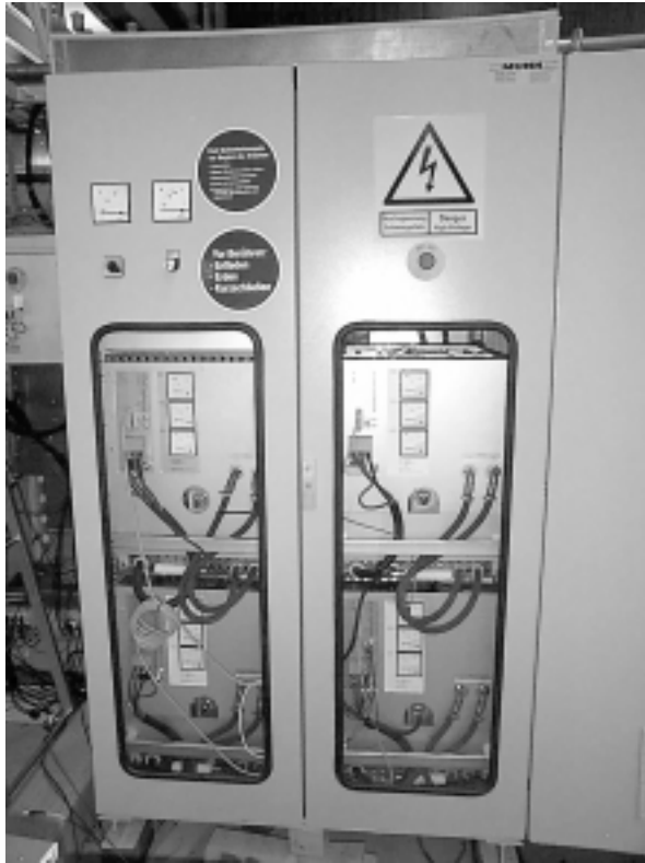
Figure 6: 300kW switch mode power supply including four 75 kW modules
