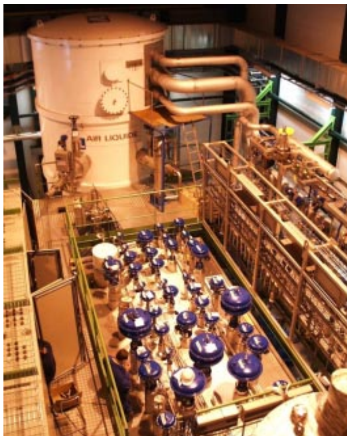
FIGURE 9. Coldbox of first 18 kW @ 4.5 K helium refrigerator
