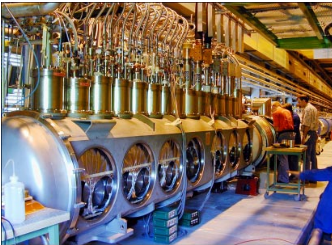
FIGURE 7. Electrical feedbox equipped with high-temperature superconductor current leads
