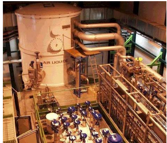
Figure 2: Coldbox of the new 18 kW refrigerator (4.5 K).
