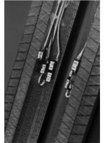
Fig. 7. Magnet coils equipped with micro-relays
