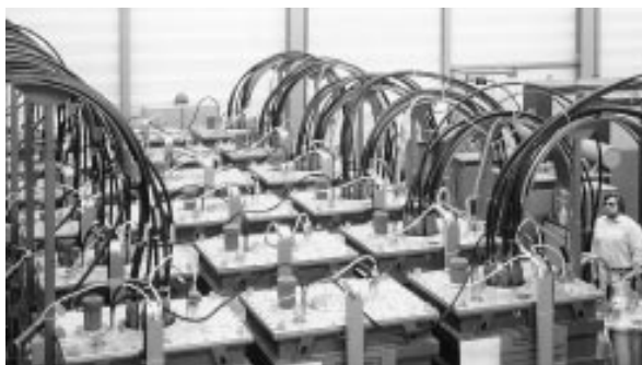
Fig. 1 Cable connections in equipment building
